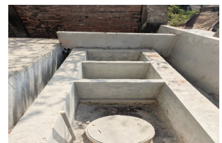
Project Name: STP for SHAHJAHAN HOMES Capacity: 12 m 3 /day Location: Police plaza concord, Hatirjheel area, Gulshan-1
