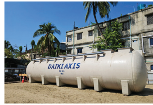
Project Name: STP for Bangladesh Fisheries Development Corporation (BFDC) Capacity: 70 m 3 /day Location: Airport Rd, Cox's Bazar, Chattogram
