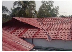
Project Name: Residential Rooftop Project Location: Gazipur bason sarak
