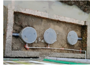
Project Name: Moheshkhali Jetty Capacity: 5 m 3 /day Location: Moheshkhali, Cox's Bazar
