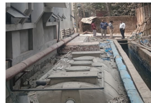
Project Name: STP for PIONEER WASHTECH Capacity: 90 m 3 /day Location: Gazipur, Dhaka
