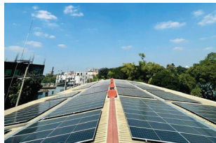
Project Name: Solar at Pioneer Wash-Tech Ltd Capacity: (1146.4 kWp DC / 1000 KW AC) Location: Nayarhat, Ashulia, Savar, Dhaka
