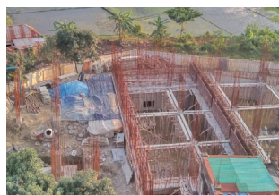
Project Name: Labib Dyeing Ltd. Capacity: 3600 m 3 /day Location: Gazipur
