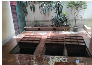
Project Name: (DNCC) Mayor's House Capacity: 10 m 3 /day Location: Sector 04, Uttara, Dhaka
