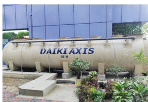
Project Name: STP for Eskayef Pharmaceuticals Limited Capacity: 40 m 3 /day Location: Tongi, Gazipur
