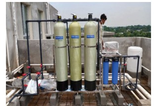
Project Name: Splash Dormitory Capacity: 1.5 m 3 /hr Location: Gazaria, Munshiganj
