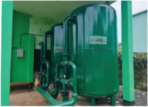
Project Name: Mirpur Cant. Swimming pool. Capacity: 30 m 3 /day Location: Mirpur 12 cant. Mirpur 12
