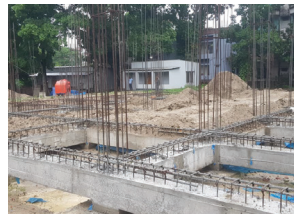
Project Name: Tangail DPHE Capacity: 750 KLD Location: Tangail
