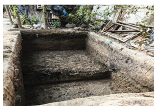
Project Name: STP for Akij Group Chairmans House Capacity: 2 m 3 /day Location: Gazipur
