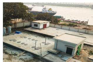
Project Name: Aligonj Govt. Housing (Zone 2) Capacity: 150 m 3 /day Location: Pagla, Narayanganj.
