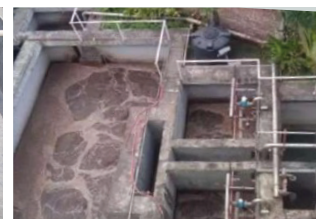
Project Name: Next Accessories Ltd. Capacity: 250 m 3 /day Location: Rupganj, Narayanganj
