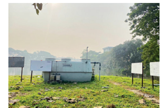
Project Name: Dhaka Cantonment Capacity: 5 m 3 /day Location: Dhaka Cantonment
