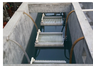
Project Name: Knit Concern Group Capacity: 2500 m 3 /day Location: Godnail, Narayanganj
