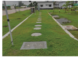
Project Name: 62 Bengal Capacity: 100 m 3 /day
