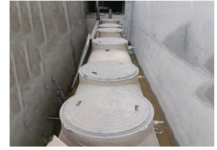
Project Name: HAssh Homes Capacity: 10 m 3 /day Location: Purbachal New Town Narayanganj
