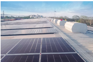
Project Name: Rooftop Solar PV System Power at Stuffing/De-Stuffing Shed Capacity: (668.5 kWp DC / 600 KW AC) Location: Mongla Port, Mongla, Bagherhat
