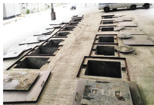
Project Name: Rab 3 Headquarter Capacity: 120 m 3 /day Location: Jheel Par, Shahjahanpur, Dhaka
