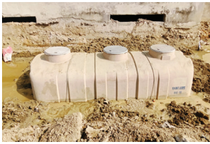
Project Name: STP for COX BAZAR FLAT PROJECT-1 Capacity: 15 m 3 /day Location: Cox bazar
