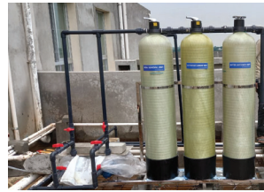
Project Name: Mana Bay Water Park (Dorm) Capacity: 1.5 m 3 /day Location: Gazaria, Munshiganj
