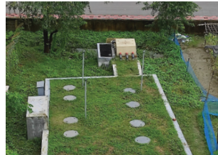
Project Name: MES Barrack Capacity: 40 m 3 /day
