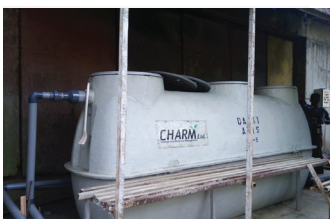
Project Name: Hotel Beach Club Capacity: 5 m 3 /day Location: Cox's Bazar
